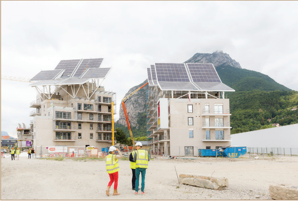
Self-sufficient building under construction in Grenoble, France, in which composites are used in the solar panels that generate energy
