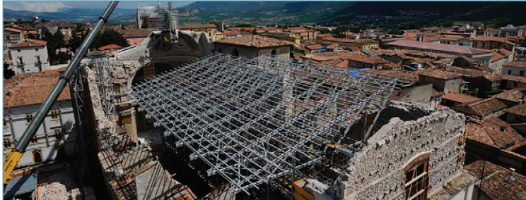
Lightweight structure designed to support a new roof after the earthquake of 2009 (S. Maria di Paganica Church, Aquila, Courtesy of Top Glass Industries)
