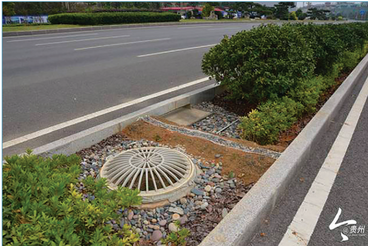
Fig. 3: Rainwater management installation near Gui'an New Area's main road (photo: Gui'an New Area Wechat account)
